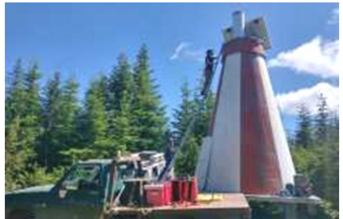
The Woss Island Trunk Repeater site
