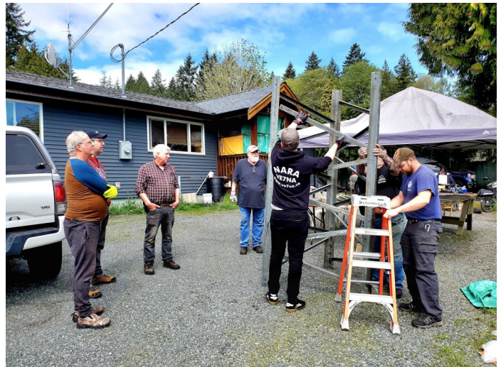
The first tower section has been completed thanks to lots of help and advice by NARA members
