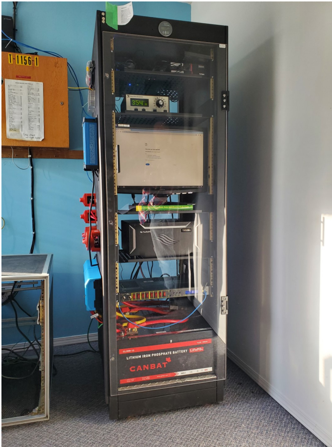
The completed rack mounted equipment and power distribution system at NARA's new station, VE7NA
