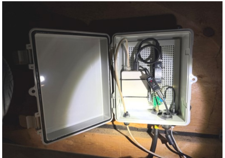
The enclosure with Raspberry Pi, SDR, and bias tee LNA power injector in a permanent location in the attic at Bruce VE7PTN’s QTH. It is installed above soffit venting for air movement; however, summertime attic temperatures can be high and may require additional heat dissipation for the Raspberry Pi to operate.
