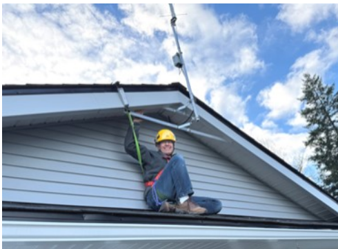
Bruce VE7PTN completing the installation of the UHF turnstile antenna at his QTH.
