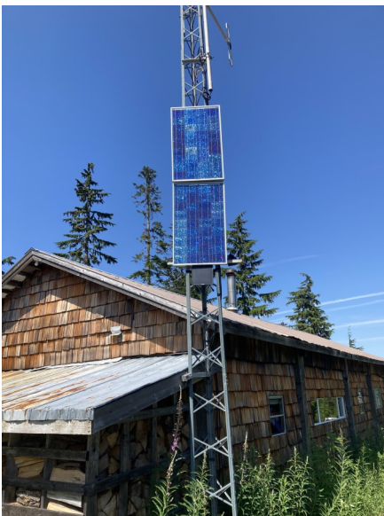
The Campbell River repeater site showing the building, solar panels, tower and antennas.
