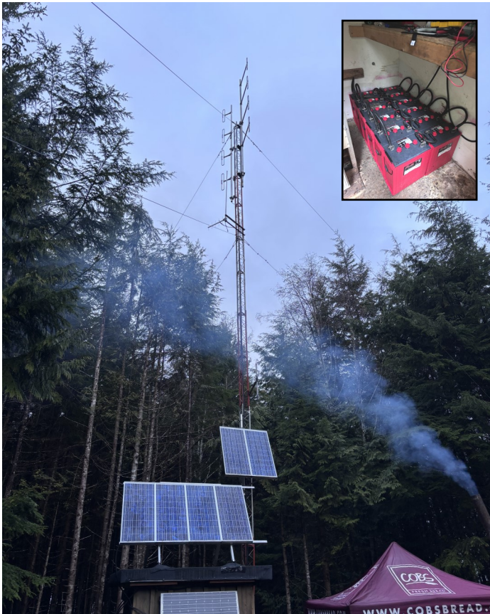
The Shelly Mountain Island Trunk System repeater site, also showing the brand new batteries in position.
