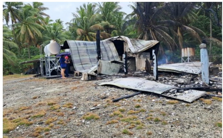
The fire at the power generator on Manihiki, North Cook Is., which essentially put the E51MWA DXpedition off the air.
